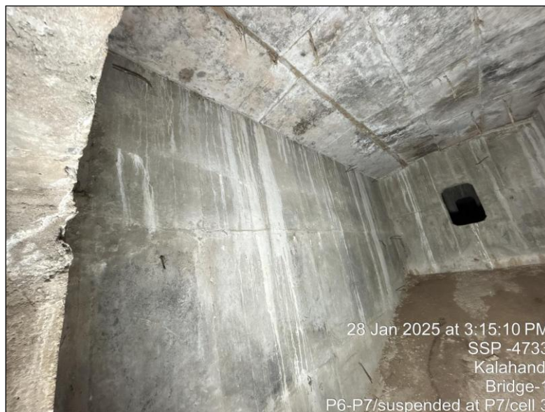
Photo 43: A view of leaching on deck slab in cell-3 (longitudinal) of Box girder in the suspended Span P6-P7 of H.L Bridge at 27/500 Km on Bhawanipatna-Khariar Road in the Kalahandi Division
