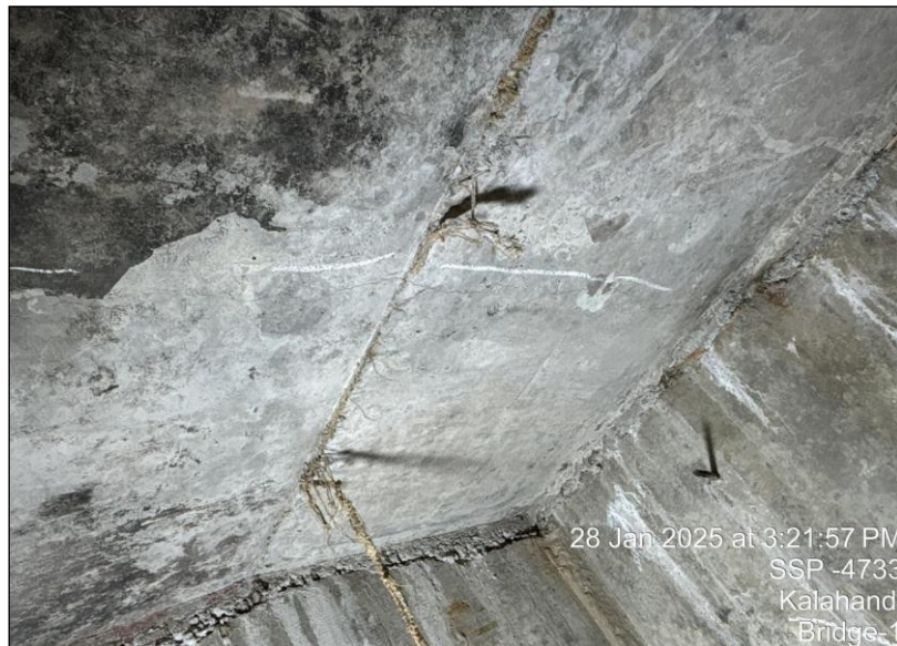
Photo 69: A view of Cracks on Deck Slab in Cell-1 in the suspended Span P7-P8 of H.L Bridge at 27/500 Km on Bhawanipatna-Khariar Road in the Kalahandi Division
