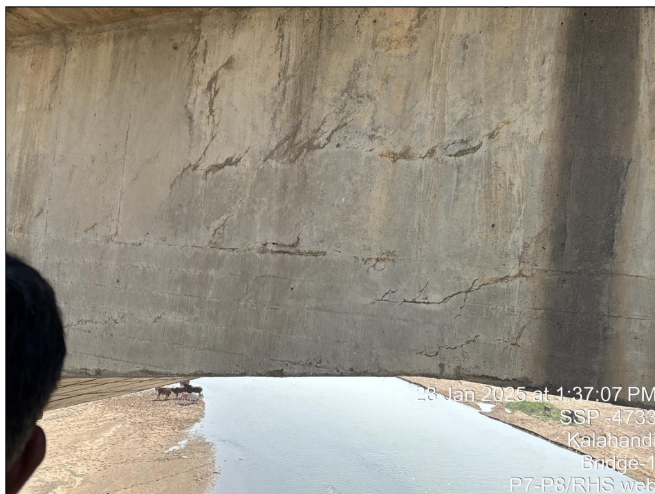
Photo 51: A view of Crack on RHS web in the Span P7-P8 of H.L Bridge at 27/500 Km on Bhawanipatna-Khariar Road in the Kalahandi Division
