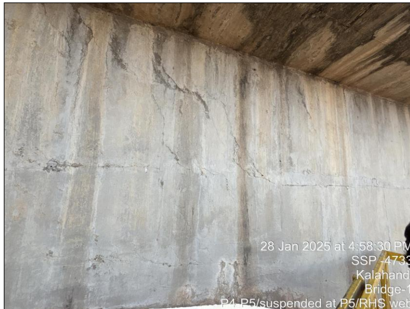
Photo 18: A view of Cracks on RHS Web near Pier P-5 in the Span P4-P5 of H.L Bridge at 27/500 Km on Bhawanipatna – Khariar Road in the Kalahandi Division.
