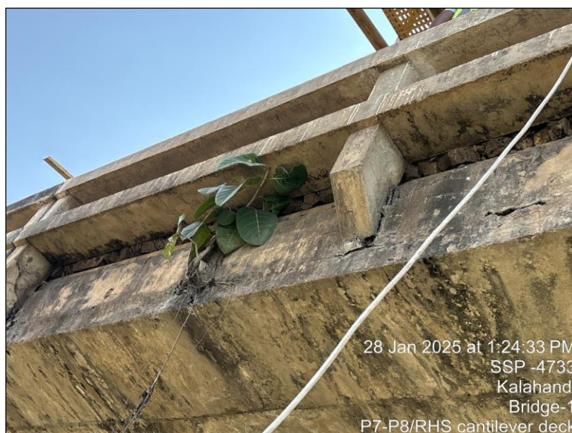
Photo 83: A view of vegetation growth on the Cantilever portion in the Span P7-P8 of H L Bridge at 27/500 Km on Bhawanipatna-Khariar Road in the Kalahandi Division.
