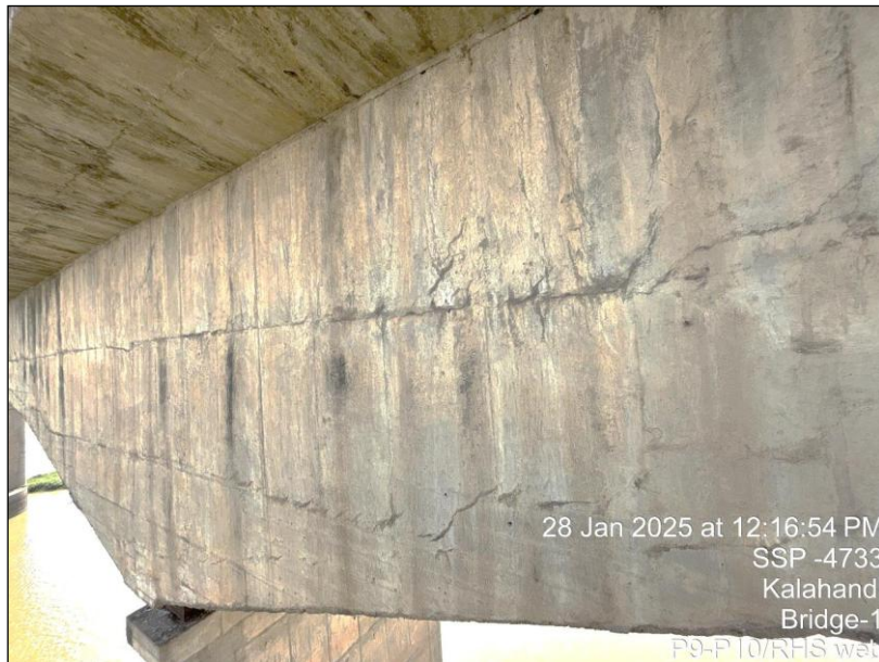
Photo 104: A view of crack on RHS web in the Span P9-P10 of H.L Bridge at 27/500 Km on Bhawanipatna-Khariar Road in the Kalahandi Division.
