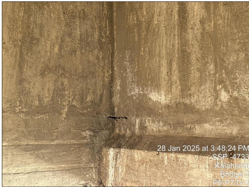
Photo 30: A view of Honeycombing on Girder-1 in the Span P6-P7 of H L Bridge at 27/500 Km on Bhawanipatna – Khariar Road in the Kalahandi Division
