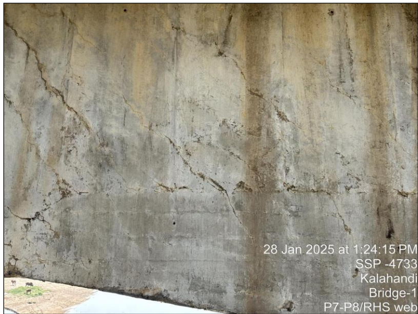
Photo 57: A view of Crack on RHS web in the Span P7-P8 of H.L Bridge at 27/500 Km on Bhawanipatna-Khariar Road in the Kalahandi Division
