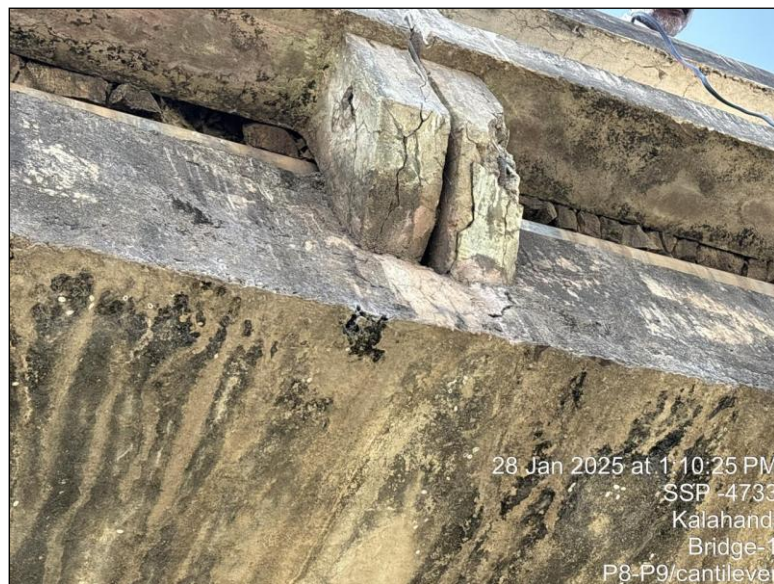
Photo 101: A view of Cracks on supporting bracket of railing in the span P8-P9 of H.L Bridge at 27/500 Km on Bhawanipatna-Khariar Road in the Kalahandi Division.
