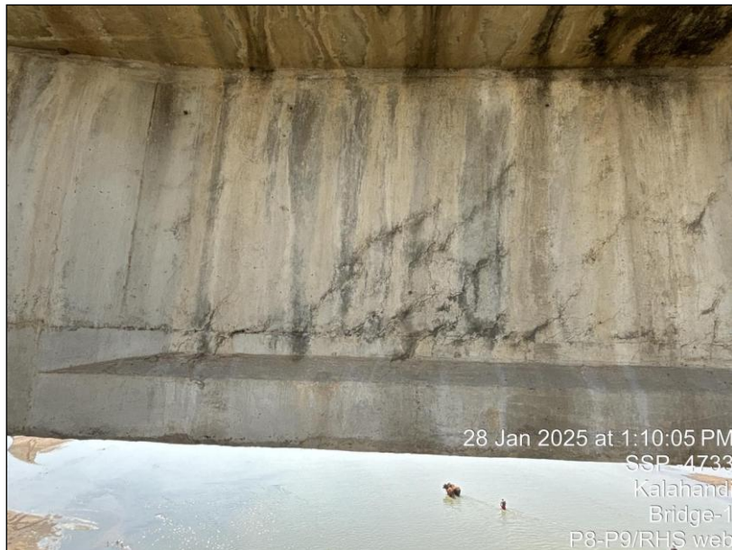
Photo 92: A view of Crack on RHS web near Pier P-8 in the Suspended Span P8-P9 of H.L Bridge at 27/500 Km on Bhawanipatna-Khariar Road in the Kalahandi Division
