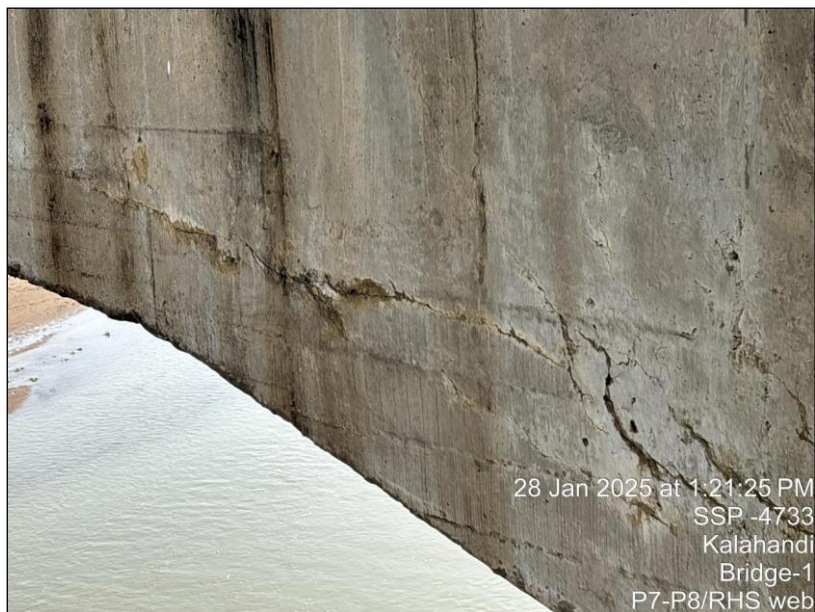
Photo 59: A view of Crack on RHS web in the Span P7-P8 of H.L Bridge at 27/500 Km on Bhawanipatna-Khariar Road in the Kalahandi Division
