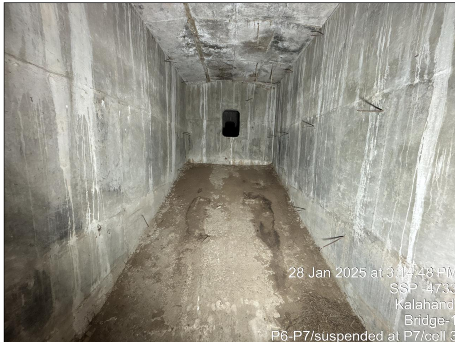
Photo 45: A view of dampness in Cell-3 (longitudinal) of Box girder in the suspended Span P6-P7 of H.L Bridge at 27/500 Km on Bhawanipatna–Khariar Road in the Kalahandi Division
