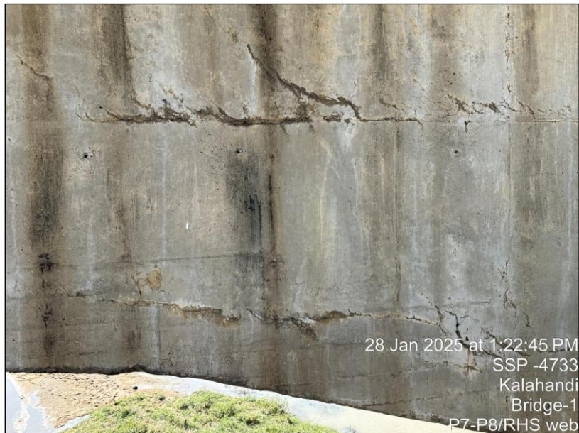
Photo 58: A view of Crack on RHS web in the Span P7-P8 of H.L Bridge at 27/500 Km on Bhawanipatna-Khariar Road in the Kalahandi Division
