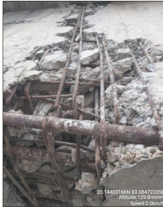
Photo 161: A view of distressed d/s soffit in the Span P11-P12 of H.L Bridge at 27/500 Km on Bhawanipatna-Khariar Road in the Kalahandi Division
