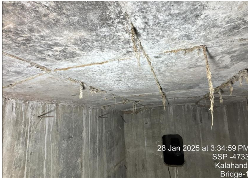
Photo 64: A view of crack on Deck Slab in Cell-1 of Box Girder near Pier P-7 in the Span P7-P8 of H.L Bridge at 27/500 Km on Bhawanipatna-Khariar Road in the Kalahandi Division
