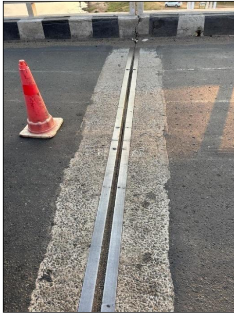
Photo 185: A view of Expansion joint fill with dust of H.L Bridge at 27/500 Km on Bhawanipatna-Khariar Road in the Kalahandi Division
