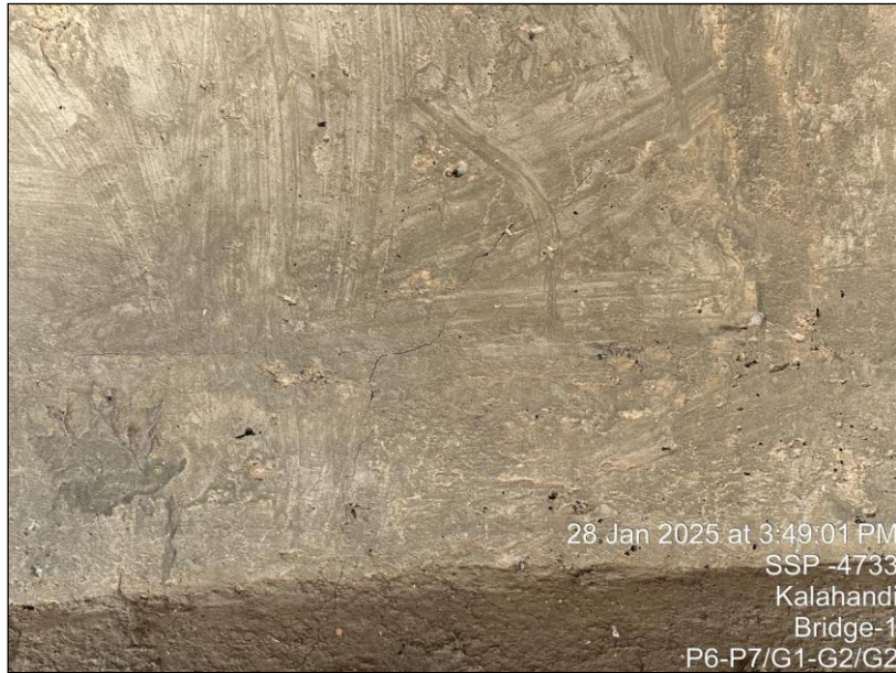
Photo 34: A view of Crack on Girder-2 in the Span P6-P7 of H.L Bridge at 27/500 Km on Bhawanipatna – Khariar Road in the Kalahandi Division
