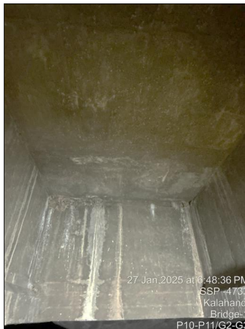
Photo 127: A view of leaching on deck slab between longitudinal girder G2-G3 in the Span P10-P11 of H.L Bridge at 27/500 Km on Bhawanipatna-Khariar Road in the Kalahandi Division.
