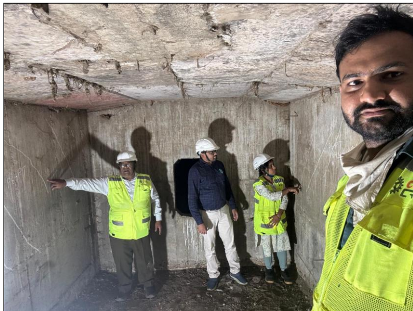
Photo 4: A view of Inspection of Crack in box Girder in span P6-P7 of H.L Bridge at 27/500 Km on Bhawanipatna – Khariar Road in the Kalahandi Division
