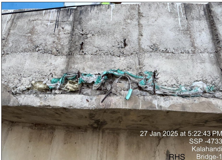
Photo 176: A view of Exposed reinforcement and Honeycombing on RHS Crash barrier in the Span P12-A2 of H.L Bridge at 27/500 Km on Bhawanipatna – Khariar Road in the Kalahandi Division.
