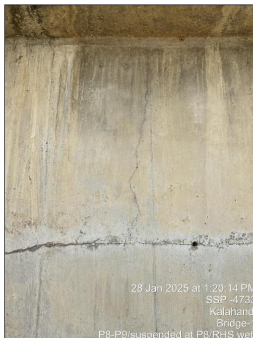
Photo 89: A view of Crack on RHS web near Pier P-8 in the Suspended Span P8-P9 of H.L Bridge at 27/500 Km on Bhawanipatna-Khariar Road in the Kalahandi Division
