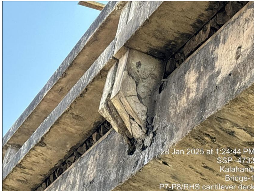
Photo 84: A view of cracks and damaged bracket of supporting railing in the RHS cantilever in the span P7-P8 of H L Bridge at 27/500 Km on Bhawanipatna-Khariar Road in the Kalahandi Division.
