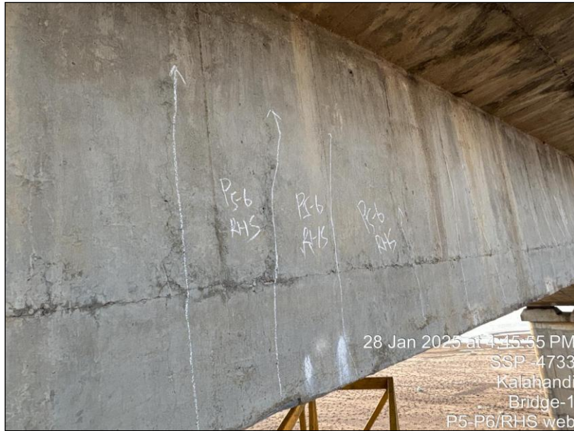
Photo 24: A view of Cracks on RHS web in the span P5-P6 of H L Bridge at 27/500 Km on Bhawanipatna – Khariar Road in the Kalahandi Division
