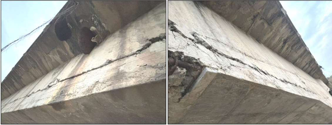
Photo 155: A view of Cracks on the distressed RHS web in the Span P11-P12 of H.L Bridge at 27/500 Km on Bhawanipatna-Khariar Road in the Kalahandi Division.
