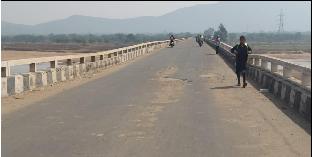
(Severe distressed Span P1-P2 as per OWD)
