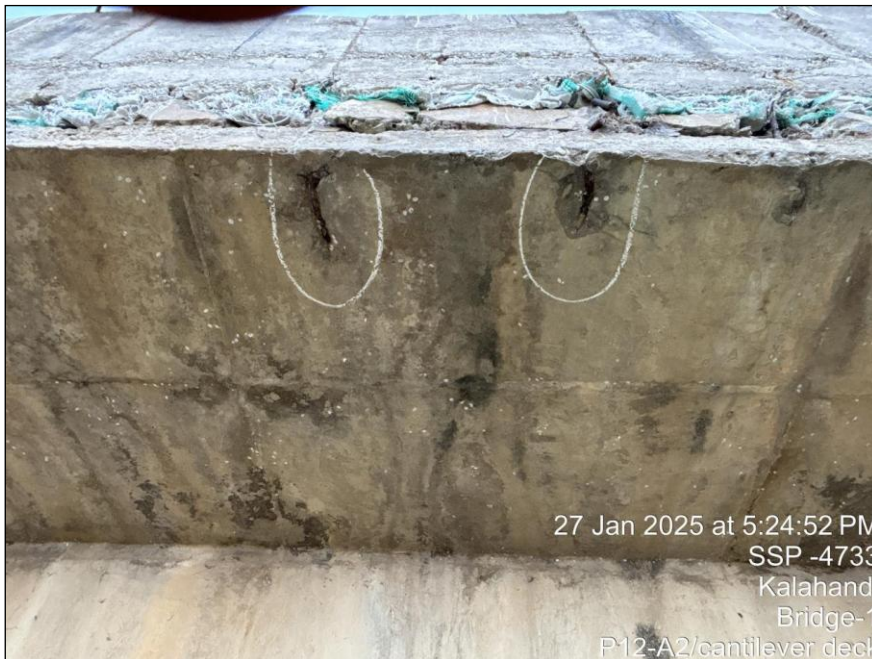
Photo 174: A view of Exposed Reinforcement at the Bottom of Cantilever Deck Slab in span P12-A2 of H.L Bridge at 27/500 Km on Bhawanipatna-Khariar Road in the Kalahandi Division.
