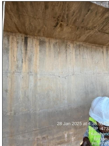
Photo 28: A view of horizontal cracks on Web at Pier P-6 in the Span P6-P7 of H L Bridge at 27/500 Km on Bhawanipatna–Khariar Road in the Kalahandi Division.
