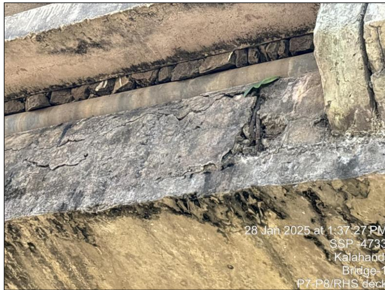
Photo 85: A view of cracks and exposed reinforcement on RHS cantilever deck Slab in the span P7-P8 of HL Bridge at 27/500 Km on Bhawanipatna-Khariar Road in the Kalahandi Division
