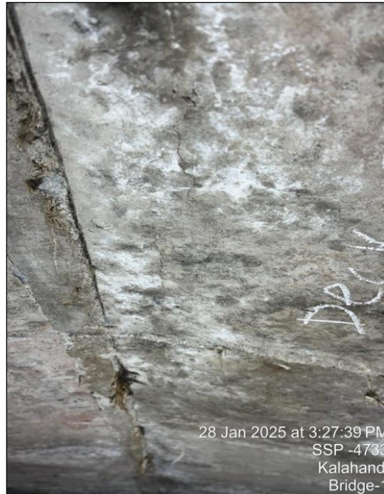
Photo 80: A view of seepage and cracks at deck Slab in cell -2 near Pier P-7 in the Span P7-P8 of H L Bridge at 27/500 Km on Bhawanipatna-Khariar Road in the Kalahandi Division .
