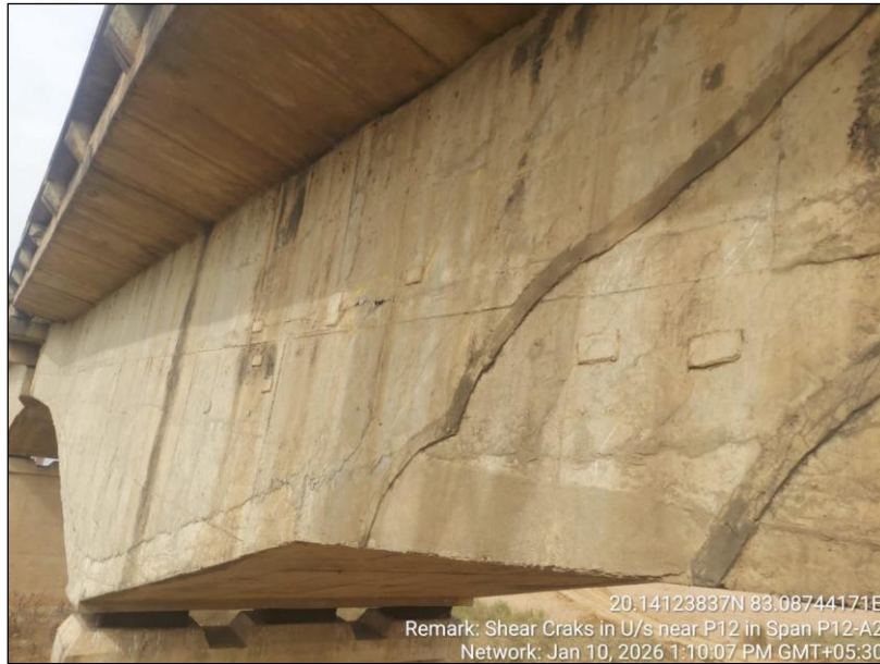
Photo 10(d): A view of Shear Cracks in U/S near Pier P-1 in the span P1-A1 of Tel Bridge of the Kalahandi Section.
