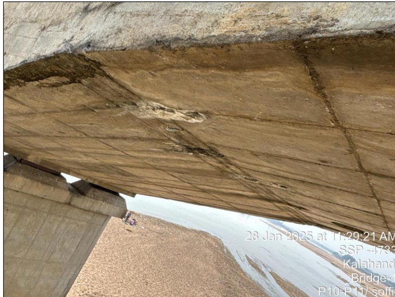
Photo 132: A view of leaching on Soffit slab in the Span P10-P11 of H.L Bridge at 27/500 Km on Bhawanipatna-Khariar Road in the Kalahandi Division
