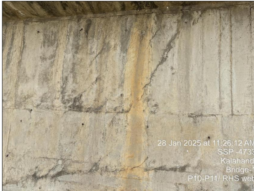
Photo 122: A view of cracks on RHS web in the Span P10-P11 of H.L Bridge at 27/500 Km on Bhawanipatna-Khariar Road in the Kalahandi Division.
