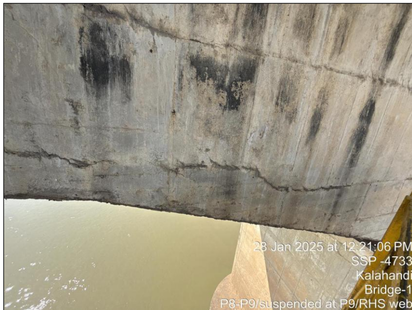
Photo 91: A view of Crack on RHS web at Pier P-9 in the Suspended Span P8-P9 of H.L Bridge at 27/500 Km on Bhawanipatna-Khariar Road in the Kalahandi Division
