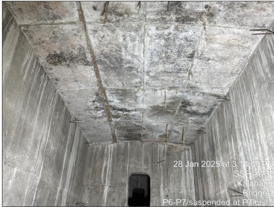
Photo 44: A view of leaching on Deck Slab in Cell-3 (longitudinal) of Box Girder in the suspended Span P6-P7 of H.L Bridge at 27/500 Km on Bhawanipatna–Khariar Road in the Kalahandi Division
