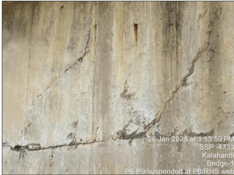
Photo 94: A view of Crack on RHS web near Pier P-8 in the Suspended Span P8-P9 of H.L Bridge at 27/500 Km on Bhawanipatna-Khariar Road in the Kalahandi Division
