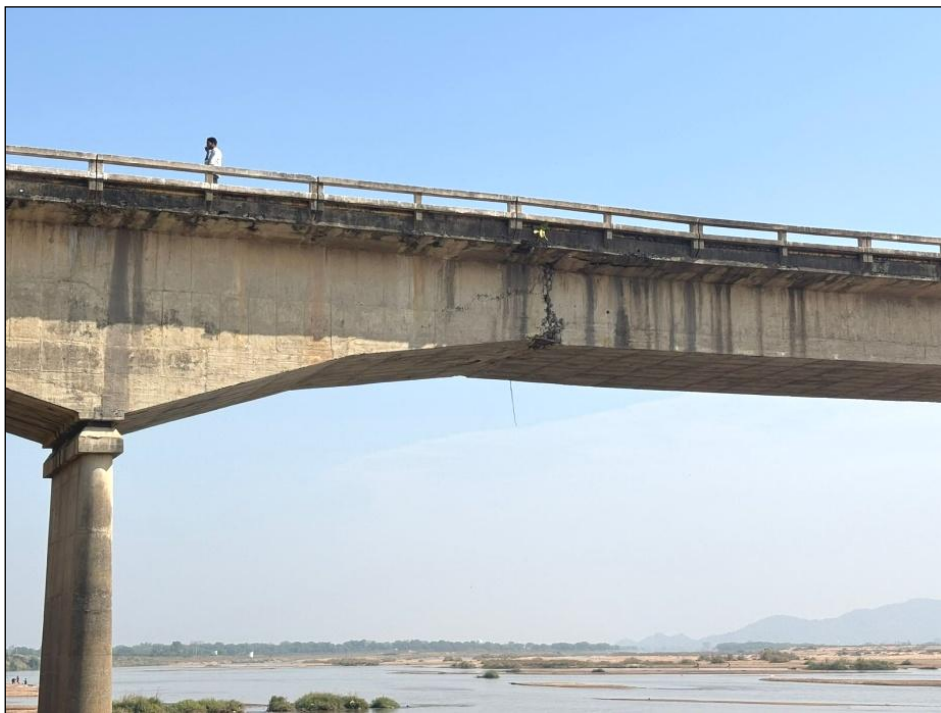
(Severe distressed Span P1-P2 as per OWD)
