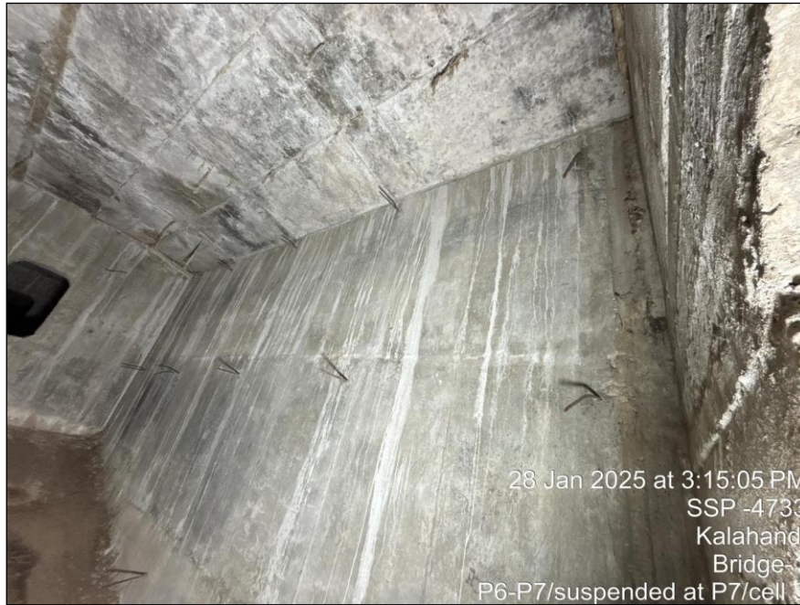
Photo 46: A view of projected reinforcement on web in cell-3 (longitudinal) of Box Girder in the Suspended Span P6-P7 of H.L Bridge at 27/500 Km on Bhawanipatna–Khariar Road in the Kalahandi Division
