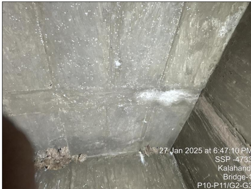
Photo 130: A view of leaching on Deck slab between girders G2-G3 in the Span P10-P11 of H.L Bridge at 27/500 Km on Bhawanipatna-Khariar Road in the Kalahandi Division.
