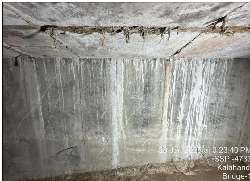
Photo 65: A view of Cracks on Middle web of Cell-1 near Pier P-7 in the Span P7-P8 of H L Bridge at 27/500 Km on Bhawanipatna-Khariar Road in the Kalahandi Division
