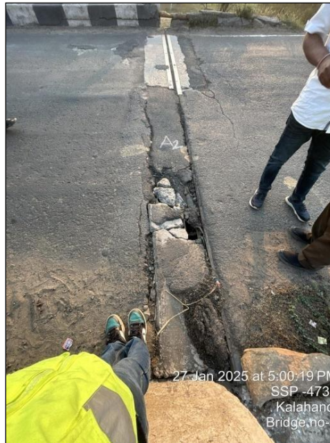
Photo 183: A view of damage Expansion joint at abutment A2 of H.L Bridge at 27/500 Km on Bhawanipatna-Khariar Road in the Kalahandi Division
