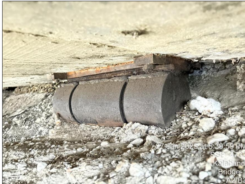
Photo 179: A view of debris accumulated near Roller-Cum-Rocker Bearing B-3 at Abutment A-2 of H.L Bridge at 27/500 Km on Bhawanipatna-Khariar Road in the Kalahandi Division
