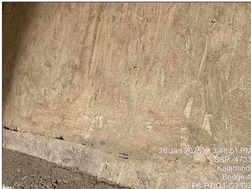
Photo 35: A view of Cracks on Girder-2 in the Span P6-P7 of H.L Bridge at 27/500 Km on Bhawanipatna – Khariar Road in the Kalahandi Division
