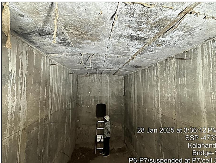
Photo 47: A view of cracks and leaching on Deck Slab in Cell-3 (longitudinal) of Box girder in the suspended Span P6-P7 of H.L Bridge at 27/500 Km on Bhawanipatna–Khariar Road in the Kalahandi Division
