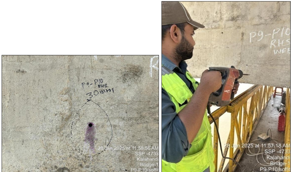
Photo 114: A view of carbonation depth measurement (30mm) on RHS Soffit in the Span P9-P10 of H L Bridge at 27/500 Km on Bhawanipatna-Khariar Road in the Kalahandi Division
