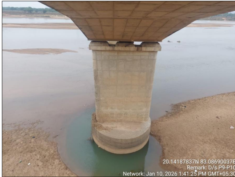
Photo 112: A view of scouring at pier P-10 in the Span P9-P10 of H.L Bridge at 27/500 Km on Bhawanipatna-Khariar Road in the Kalahandi Division
