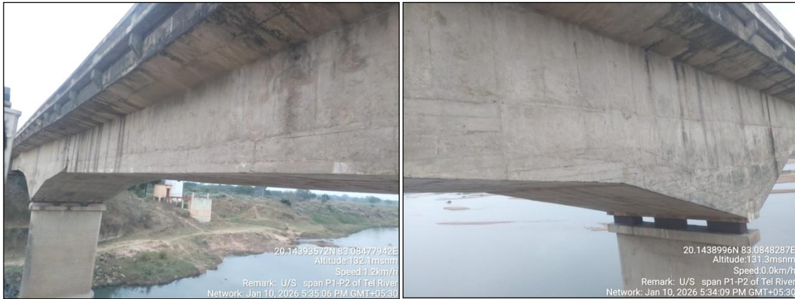
Photo 157: A LHS (u/s) view of distressed Span P11-P12 of H.L Bridge at 27/500 Km on Bhawanipatna-Khariar Road in the Kalahandi Division.
