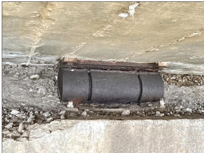
Photo 178: A view of debris accumulate near Roller-Cum-Rocker Bearing B-2 at Abutment A-2 of H.L Bridge at 27/500 Km on Bhawanipatna-Khariar Road in the Kalahandi Division.
