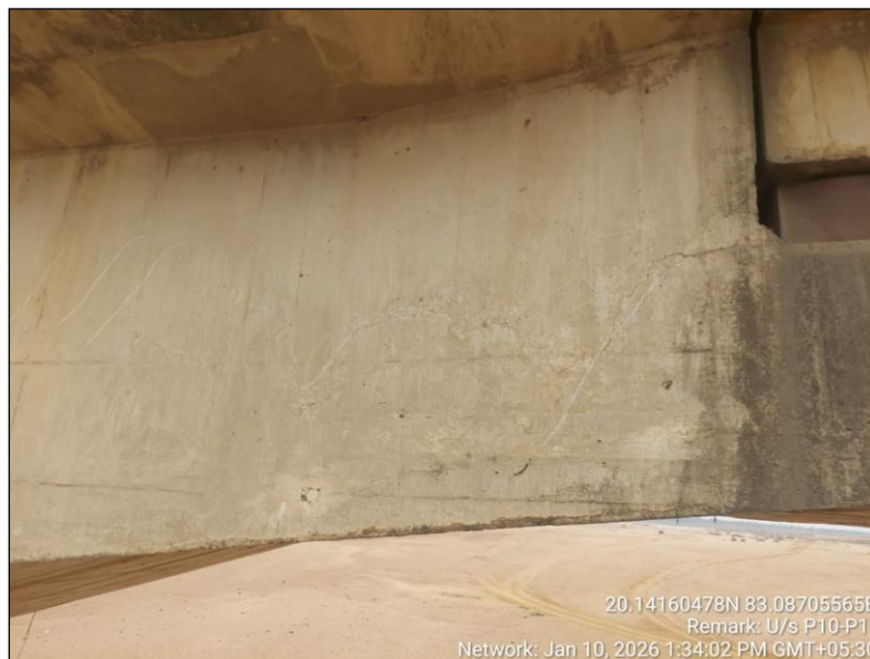
Photo 15: A view of cracks on web near articulation in the Span P2-P3 of H.L Bridge at 27/500 Km on Bhawanipatna–Khariar Road in the Kalahandi Division
