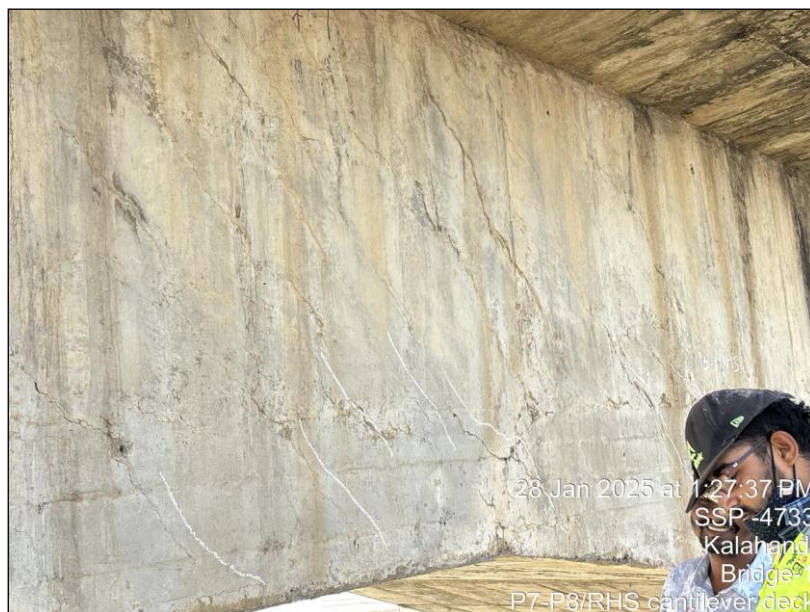
Photo 53: A view of Crack on RHS web in the Span P7-P8 of H.L Bridge at 27/500 Km on Bhawanipatna-Khariar Road in the Kalahandi Division
