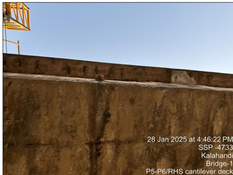
Photo 27: A view of cracks and exposed reinforcement and seepage through drainage spout on cantilever deck slab in the Span P5-P6 of H.L Bridge at 27/500 Km on Bhawanipatna – Khariar Road in the Kalahandi Division.
