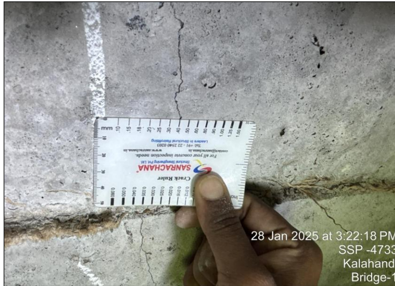
Photo 68: A view of crack width measurement (0.40 mm) on Deck Slab in Cell-1 in the Span P7-P8 of H L Bridge at 27/500 Km on Bhawanipatna-Khariar Road in the Kalahandi Division
