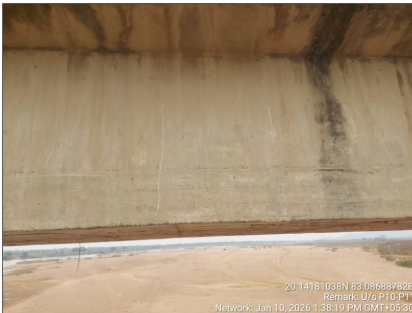
Photo 14(b): A view of cracks on the web (u/s) in the Span P2-P3 of H.L Bridge at 27/500 Km on Bhawanipatna–Khariar Road in the Kalahandi Division.
