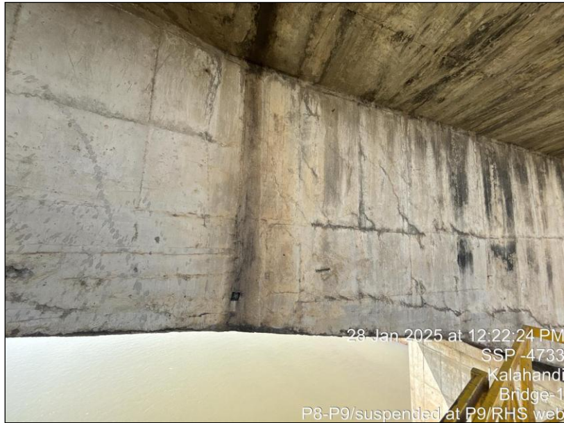
Photo 90: A view of Crack on RHS web near Pier P-9 in the Suspended Span P8-P9 of H.L Bridge at 27/500 Km on Bhawanipatna-Khariar Road in the Kalahandi Division
