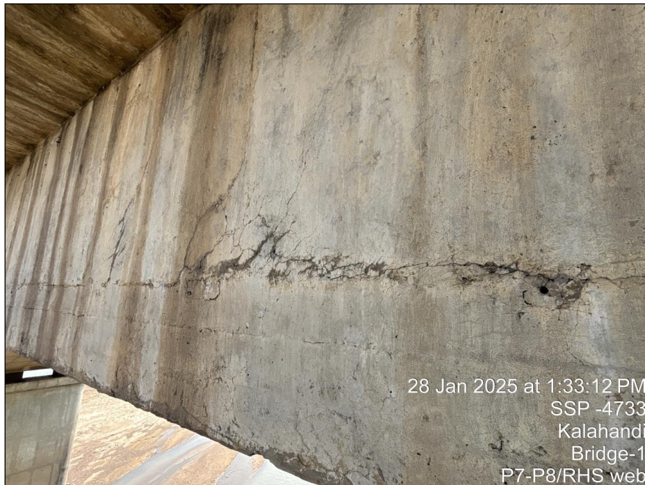
Photo 52: A view of Crack on RHS web in the Span P7-P8 of H.L Bridge at 27/500 Km on Bhawanipatna-Khariar Road in the Kalahandi Division
