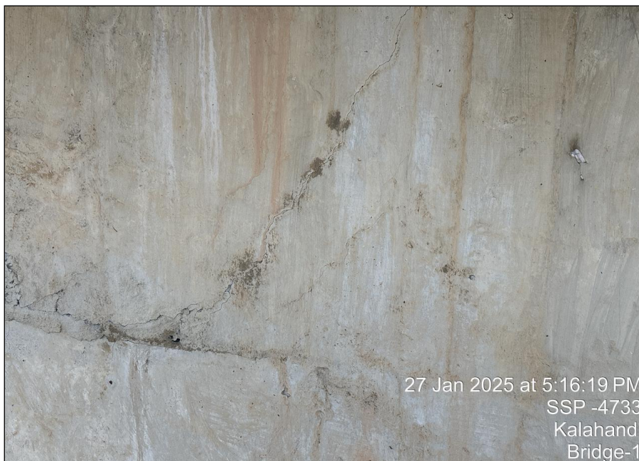
Photo 172: A view of Crack on RHS web in the Span P12-A2 of H.L Bridge at 27/500 Km on Bhawanipatna – Khariar Road in the Kalahandi Division.
