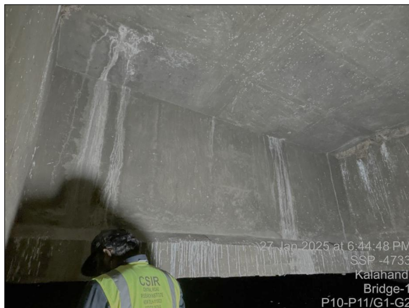
Photo 125: A view of leaching on deck slab between girders G1-G2 in the Span P10-P11 of H.L Bridge at 27/500 Km on Bhawanipatna-Khariar Road in the Kalahandi Division.
