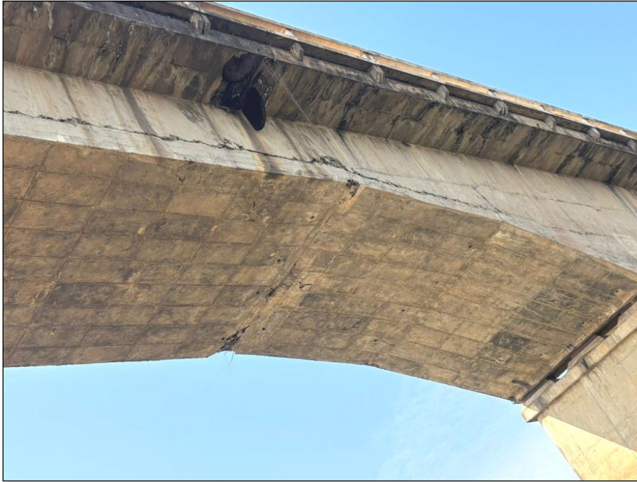
(Severe distressed Span P1-P2 as per OWD)
