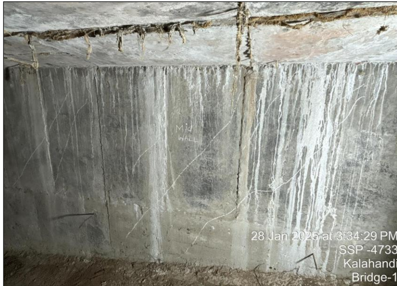
Photo 62: A General view of cracks on Middle wall of Cell-1 near Pier P-7 in the Span P7-P8 of H.L Bridge at 27/500 Km on Bhawanipatna–Khariar Road in the Kalahandi Division
