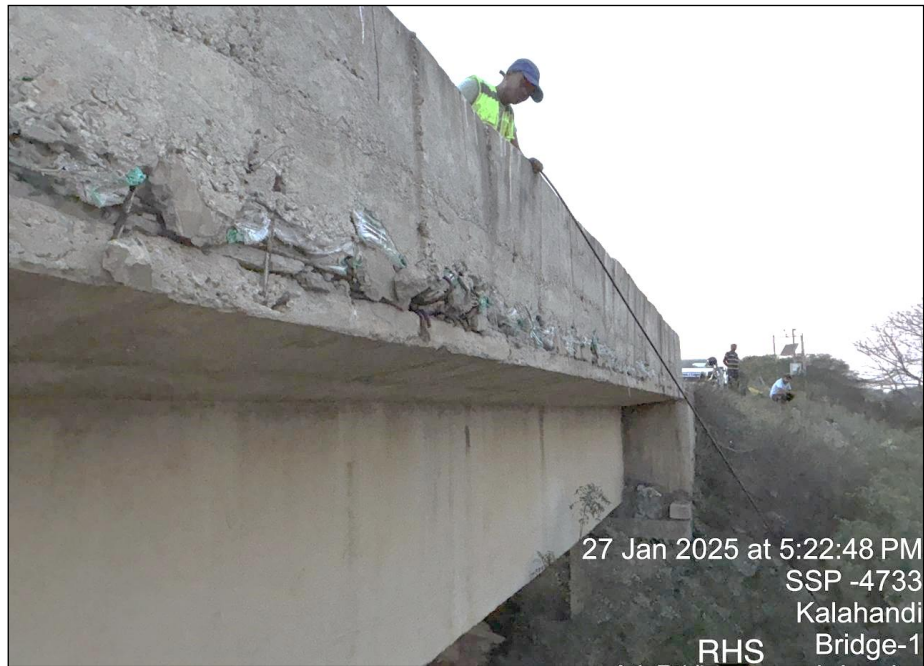
Photo 175: A view of Exposed reinforcement and Honeycombing on Crash barrier in the Span P12-A2 of H.L Bridge at 27/500 Km on Bhawanipatna–Khariar Road in the Kalahandi Division.
