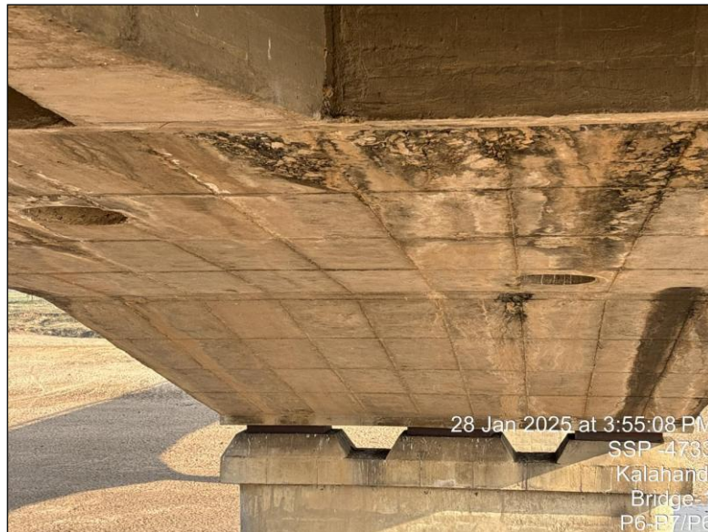
Photo 49: A view of seepage on Deck Slab at Pier P-6 in Span P6-P7 of H.L. Bridge at 27/500 Km on Bhawanipatna-Khariar Road in the Kalahandi Division.
