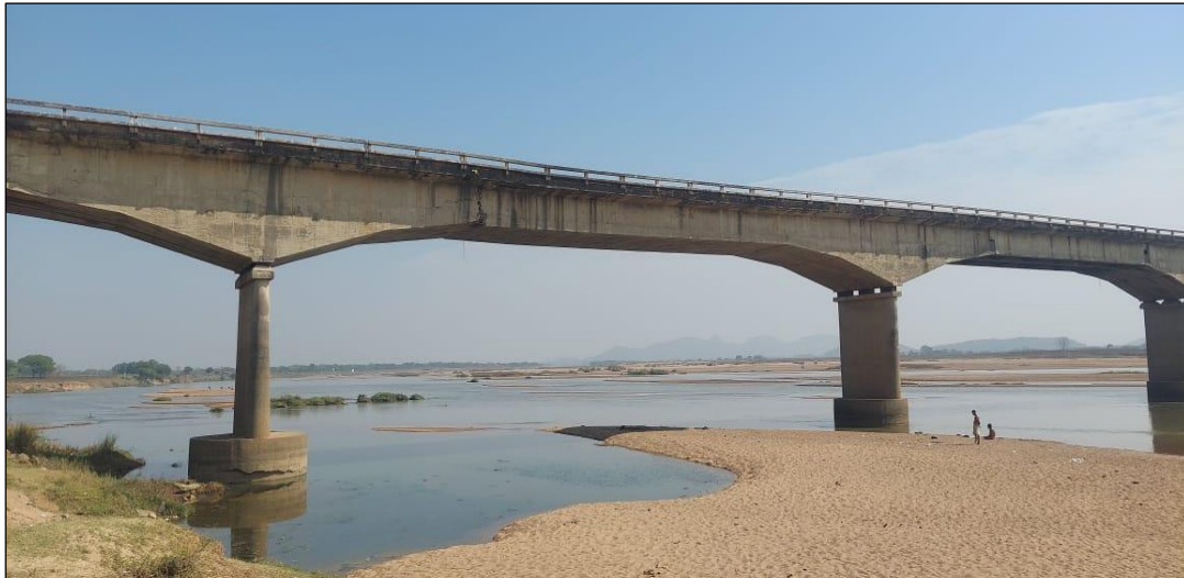
(Severe distressed Span P1-P2 as per OWD)
