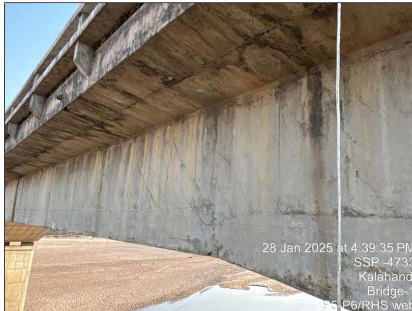
Photo 22: A view of cracks on RHS Web in the span P-5-P6 of H.L Bridge at 27/500 Km on Bhawanipatna – Khariar Road in the Kalahandi Division.
