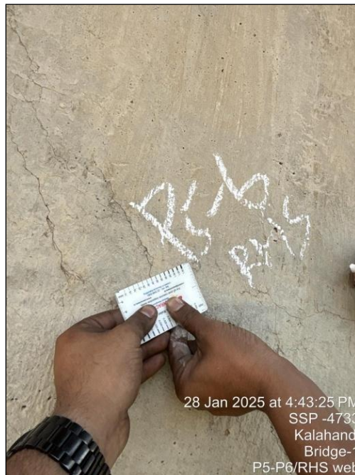
Photo 25: A view of crack width measurement (0.40mm) on RHS web in the span P5-P6 of H.L Bridge at Km 27/500 on Bhawanipatna – Khariar Road in the Kalahandi Division.
