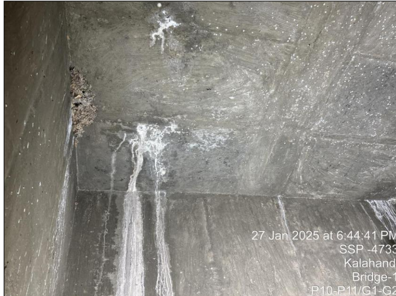
Photo 129: A view of leaching on Deck slab between girders G1-2 in the Span P10-P11 of H.L Bridge at 27/500 Km on Bhawanipatna-Khariar Road in the Kalahandi Division.
