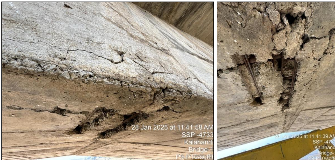
Photo 111: A view of cracks and Exposed Reinforcement on soffit slab in the Span P9-P10 of H.L Bridge at 27/500 Km on Bhawanipatna-Khariar Road in the Kalahandi Division
