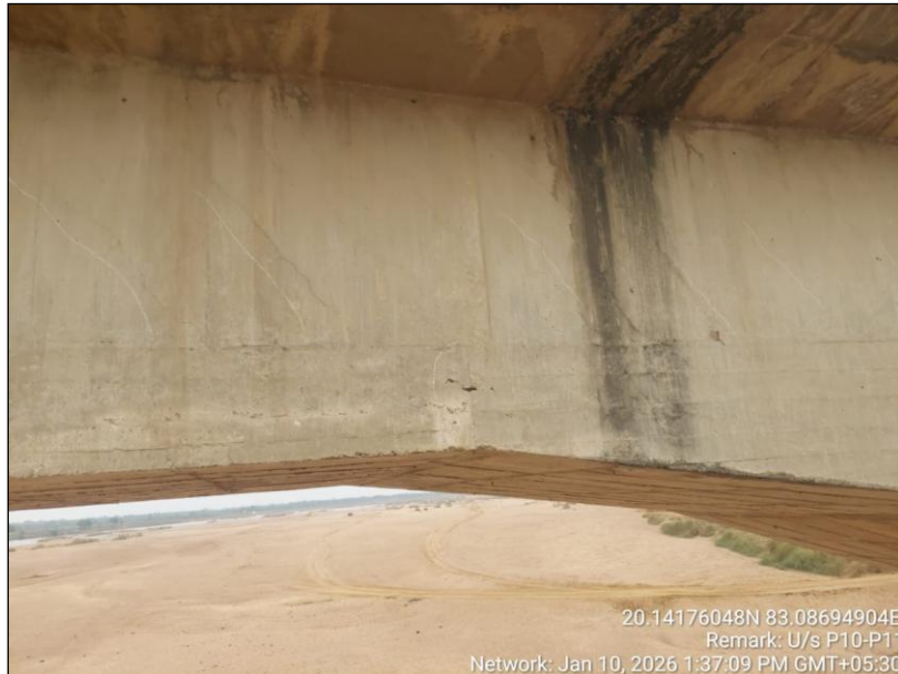
Photo 14(c): A view of cracks on web in the Span P2-P3 of H.L Bridge at 27/500 Km on Bhawanipatna–Khariar Road in the Kalahandi Division
