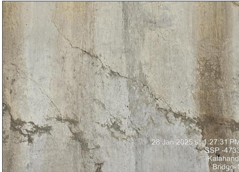
Photo 54: A view of Crack on RHS web in the Span P7-P8 of H.L Bridge at 27/500 Km on Bhawanipatna-Khariar Road in the Kalahandi Division
