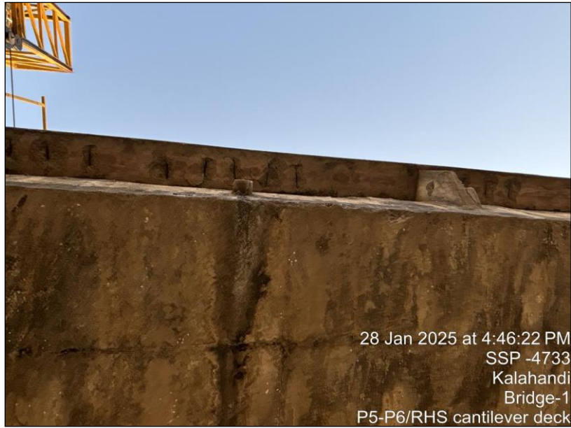
Photo 190: A typical view of drainage spout of H.L Bridge at 27/500 Km on Bhawanipatna-Khariar Road in the Kalahandi Division
