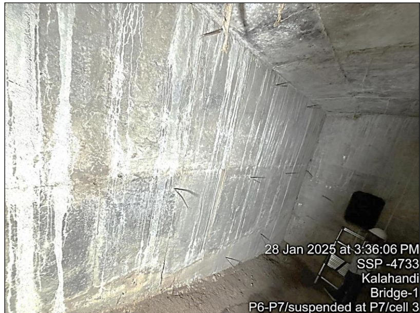
Photo 48: A General view of projected reinforcement on RHS wall of Cell-3 (longitudinal) in the suspended Span P6-P7 of H.L. Bridge at 27/500 Km on Bhawanipatna–Khariar Road in the Kalahandi Division
