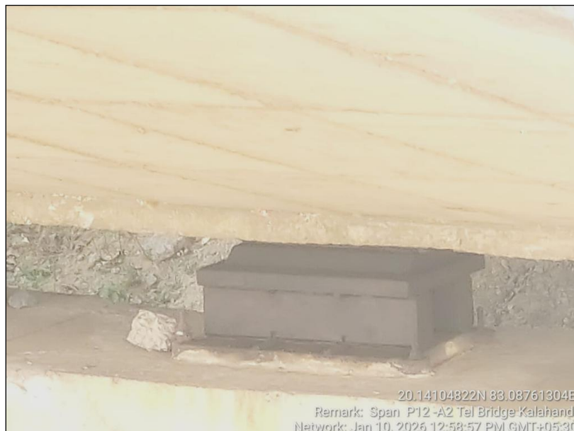
Photo 9(c): A view of Missing Tie plates in the Rocker-cum-cut Roller bearings at Abutment A-1 in the Tel Bridge of the Kalahandi Section.
