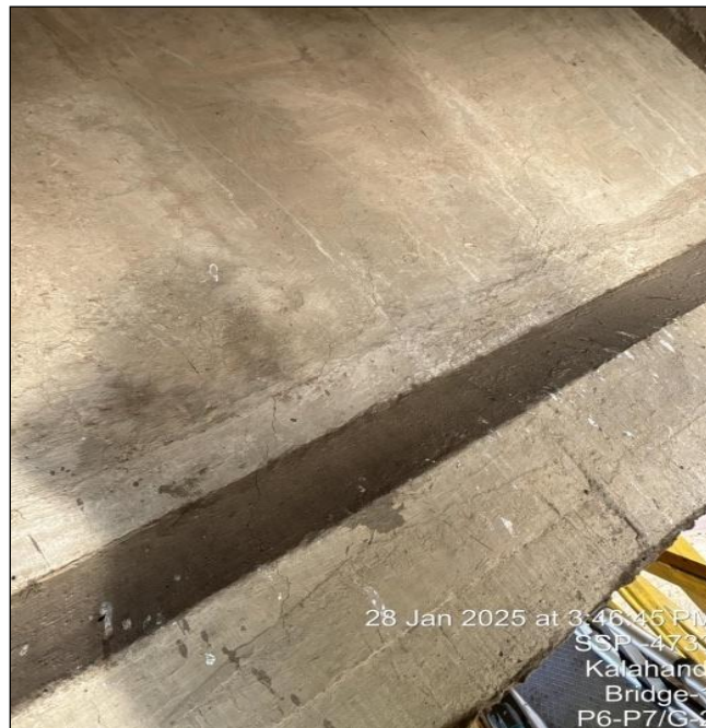
Photo 33: A view of Cracks on Girder-2 in the Span P6-P7 of H.L Bridge at 27/500 Km on Bhawanipatna – Khariar Road in the Kalahandi Division
