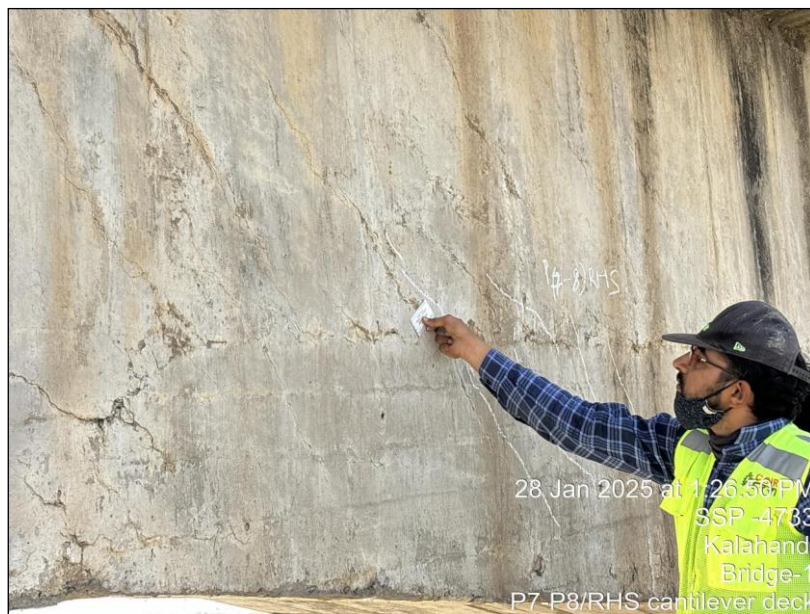
Photo 55: A view of Crack width measurement on RHS web in the Span P7-P8 of HL Bridge at 27/500 Km on Bhawanipatna-Khariar Road in the Kalahandi Division
