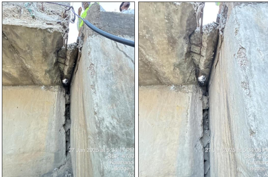
Photo 182: A view of Expansion joint and Exposed Reinforcement near Abutment A-2 of H.L Bridge at 27/500 Km on Bhawanipatna-Khariar Road in the Kalahandi Division.
