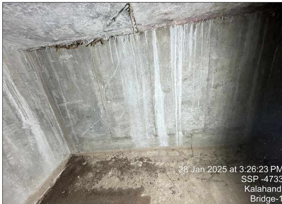
Photo 71: A view of Cracks on mid wall in Cell-2 near Pier P-7 in the Span P7-P8 of H.L Bridge at 27/500 Km on Bhawanipatna-Khariar Road in the Kalahandi Division
