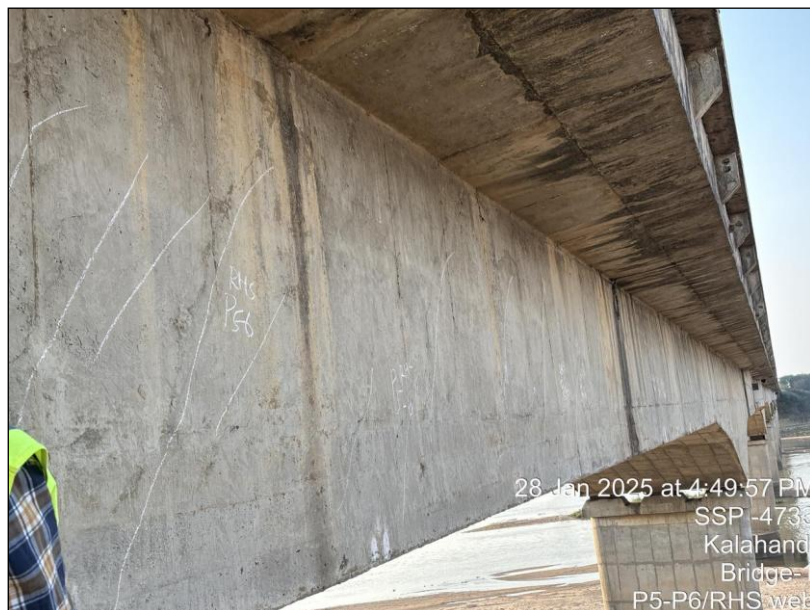
Photo 23: A view of Cracks on RHS web in the span P5-P6 of H L Bridge at 27/500 Km on Bhawanipatna–Khariar Road in the Kalahandi Division.
