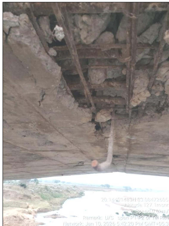
Photo: 162: A view of distressed soffit in the Span P11-P12 of H.L Bridge at 27/500 Km on Bhawanipatna-Khariar Road in the Kalahandi Division
