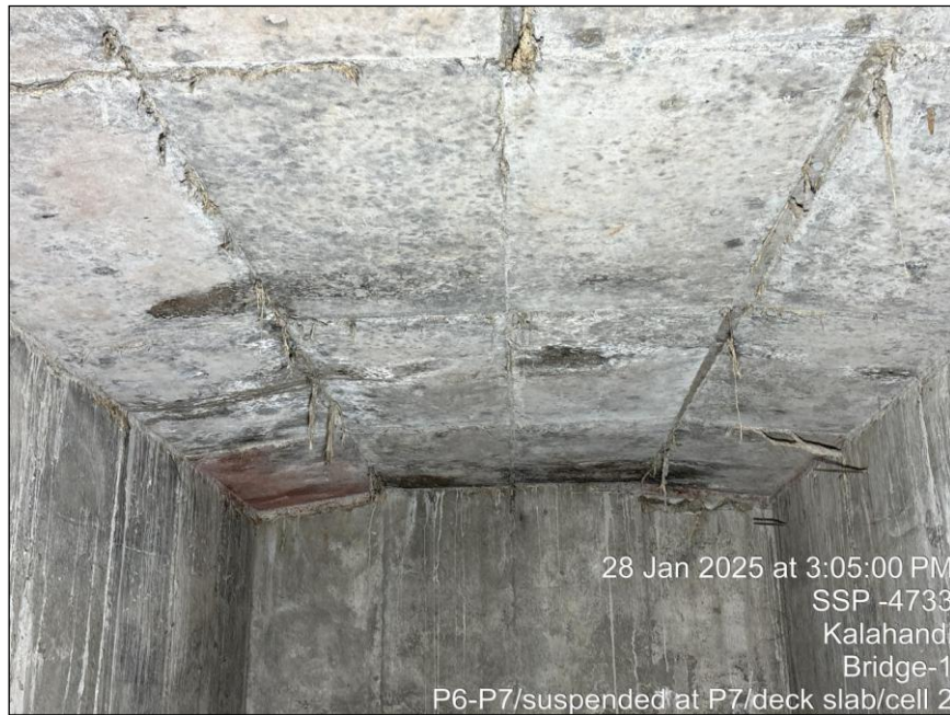
Photo 42: A view of leaching on Deck Slab in Cell-2 near Pier P-7 of Box girder in the Suspended Span P6-P7 of H.L Bridge at 27/500 Km on Bhawanipatna-Khariar Road in the Kalahandi Division.
