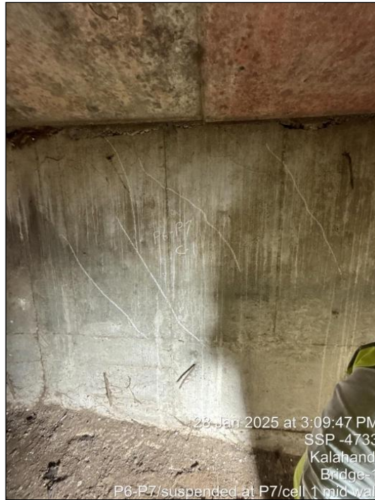
Photo 40: A view of Cracks on middle web in cell-1 near Pier P-7 in the Span P6-P7 of H.L Bridge at 27/500 Km on Bhawanipatna–Khariar Road in the Kalahandi Division
