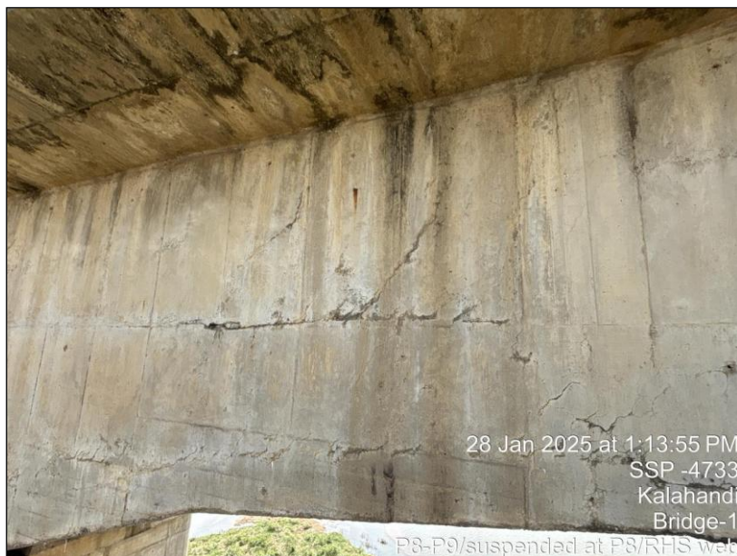
Photo 93: A view of Crack on RHS web near Pier P-8 in the Suspended Span P8-P9 of H.L Bridge at 27/500 Km on Bhawanipatna-Khariar Road in the Kalahandi Division
