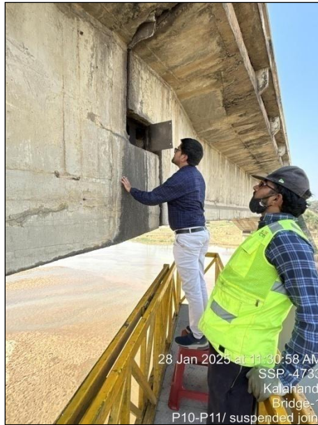
Photo 187: A typical view of leakage through Expansion joint of H.L Bridge at Km 27/500 on Bhawanipatna-Khariar Road in the Kalahandi Division
