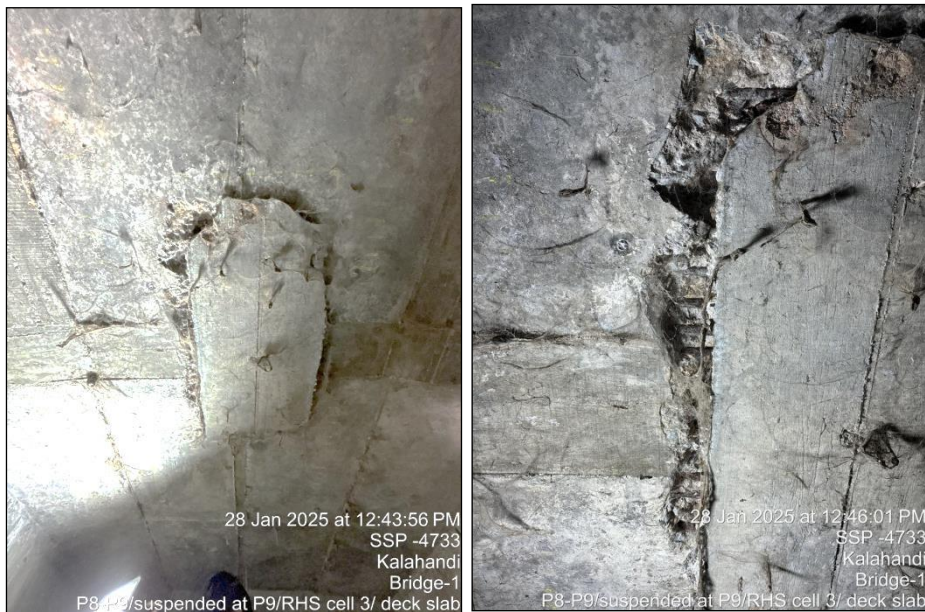
Photo 95: A view of Patch repair and exposed reinforcement on Deck Slab in RHS cell-3 near Pier P-9 in the Span P8-P9 of H.L Bridge at 27/500 Km on Bhawanipatna-Khariar Road in the Kalahandi Division.
