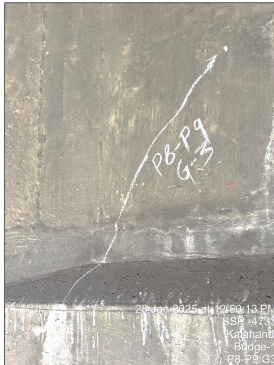
Photo 88: A view of Crack on Girder G-3 at Pier P-8 in the Suspended Span P8-P9 of H L Bridge at 27/500 Km on Bhawanipatna-Khariar Road in the Kalahandi Division.
