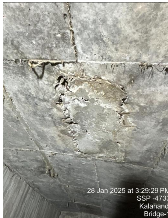
Photo 79: A view of repaired shear punching of Deck Slab in cell-2 near Pier P-7 in the Span P7-P8 of H.L Bridge at 27/500 Km on Bhawanipatna-Khariar Road in the Kalahandi Division
