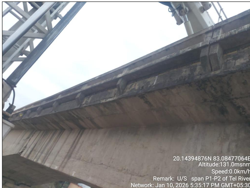
Photo 156: A LHS (u/s) view of cantilever deck slab of distressed Span P11-P12 of H.L Bridge at 27/500 Km on Bhawanipatna-Khariar Road in the Kalahandi Division
