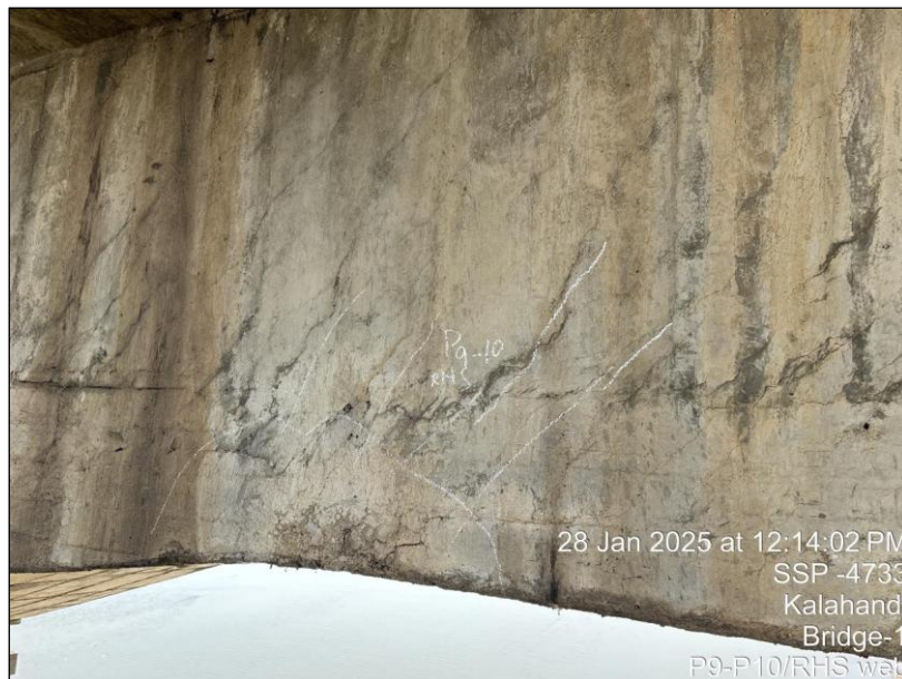
Photo 107: A view of crack on RHS web in the Span P9-P10 of H.L Bridge at 27/500 Km on Bhawanipatna-Khariar Road in the Kalahandi Division
