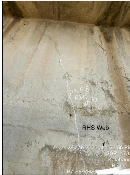
Photo 60: A view of 0.50mm Crack on RHS web in the Span P7-P8 of H L Bridge at 27/500 Km on Bhawanipatna-Khariar Road in the Kalahandi Division
