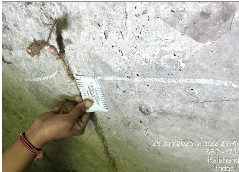
Photo 67: A view of crack width measurement (0.40 mm) on Deck Slab of Cell-1 near Pier P-7 in the Span P7-P8 of H.L Bridge at 27/500 Km on Bhawanipatna-Khariar Road in the Kalahandi Division
