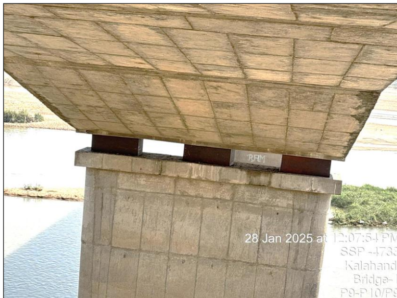
Photo 103: A view of bottom surface of girder near Pier P-9 in the Span P9-P10 of H.L Bridge at 27/500 Km on Bhawanipatna-Khariar Road in the Kalahandi Division.
